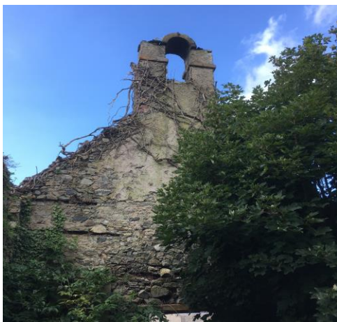
The church belltower which is in danger of collapse
