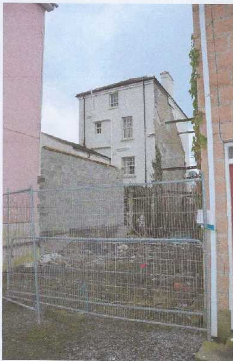
View of rear 12 St Peter's Street, rubblestone wall (ivy) to yard, proposed building extent in approximate position of Heras fencing. Blockwork wall indicates rear of ongoing 3 storey development.
