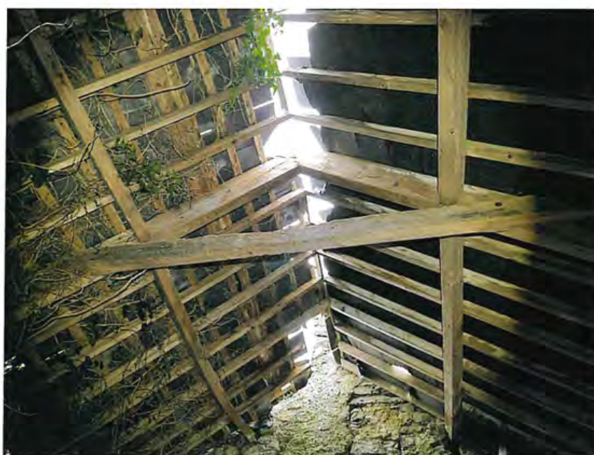
Figure 15.0 Byre roof damage
