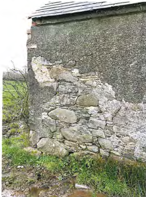
Figure 10.0 Cracking at north end of rear elevation
