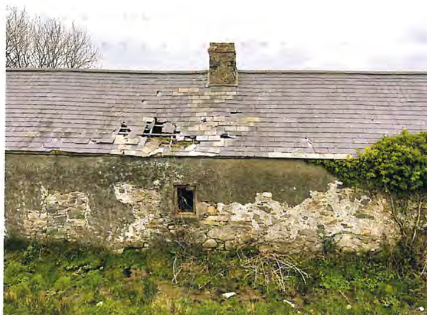
Figure 4.0 Localised loss of slates on rear slope
