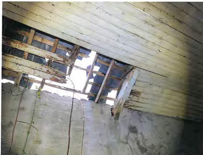
Figure 14.0 Failed truss end and rafter tails
