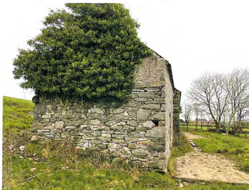
Figure 9.0 Ivy growth on byre gable
