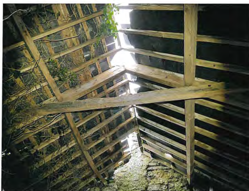
Figure 15.0 Byre roof damage
