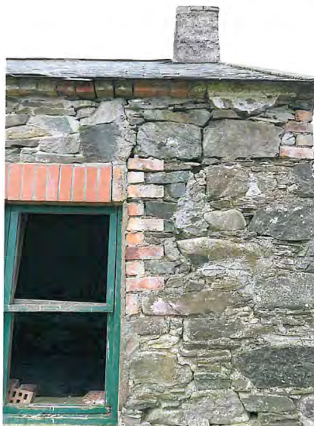
Figure 6.0 Run of near-vertical cracking (to right of window)
