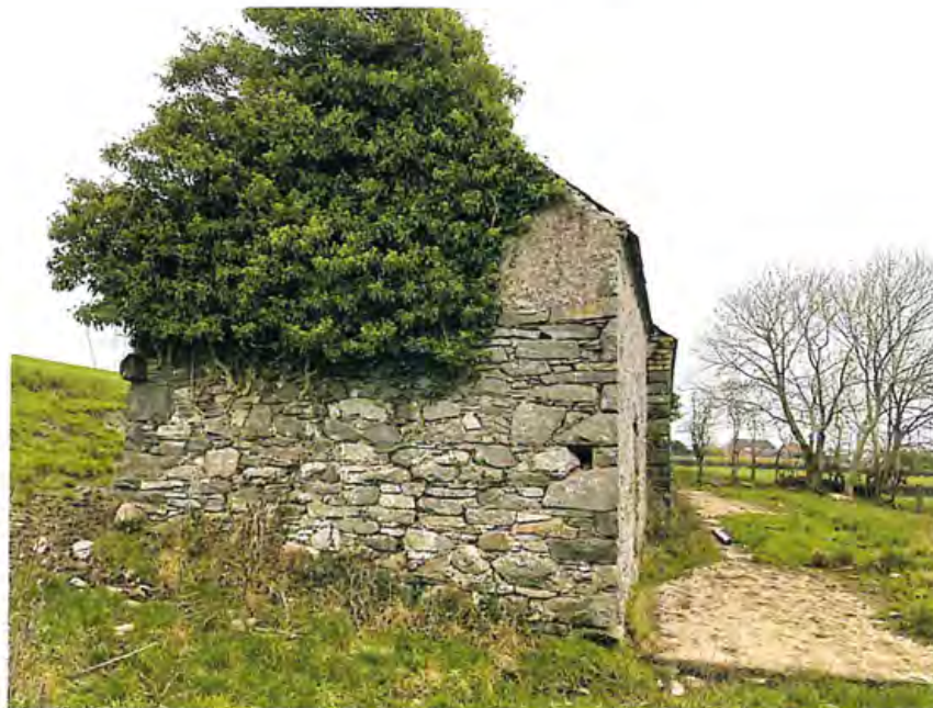
Figure 9.0 Ivy growth on byre gable
