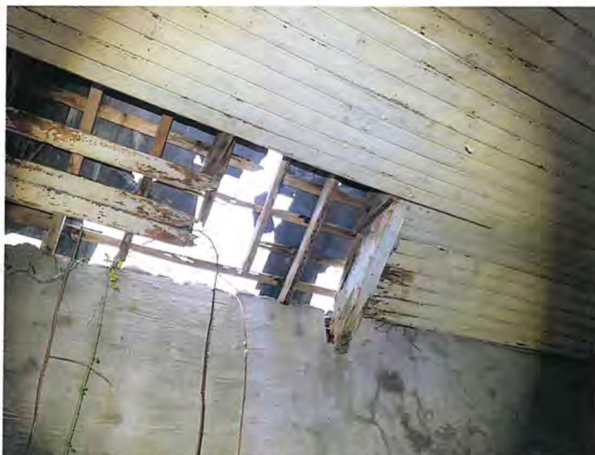
Figure 14.0 Failed truss end and rafter tails
