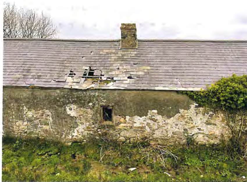
Figure 4.0 Localised loss of slates on rear slope
