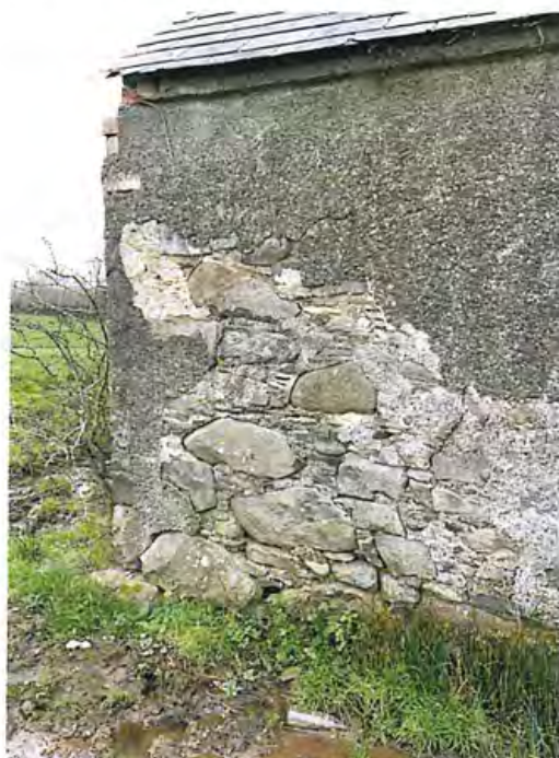
Figure 10.0 Cracking at north end of rear elevation
