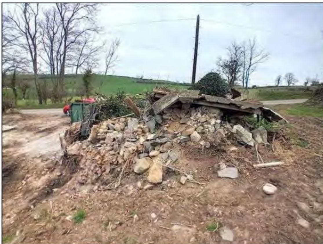
Figure 6- Collapsed eastern elevation
