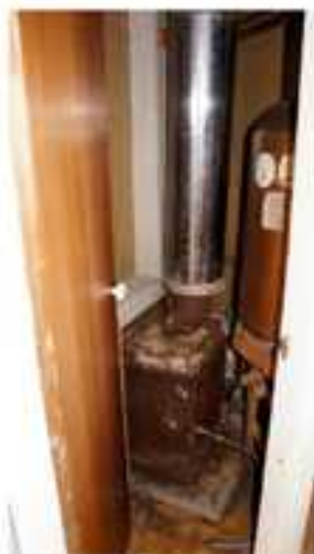
Central heating boiler
