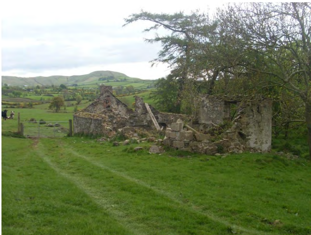
Approach to the dwelling which is clearly not 'substantially intact' as per the SPPS and CTY 3
