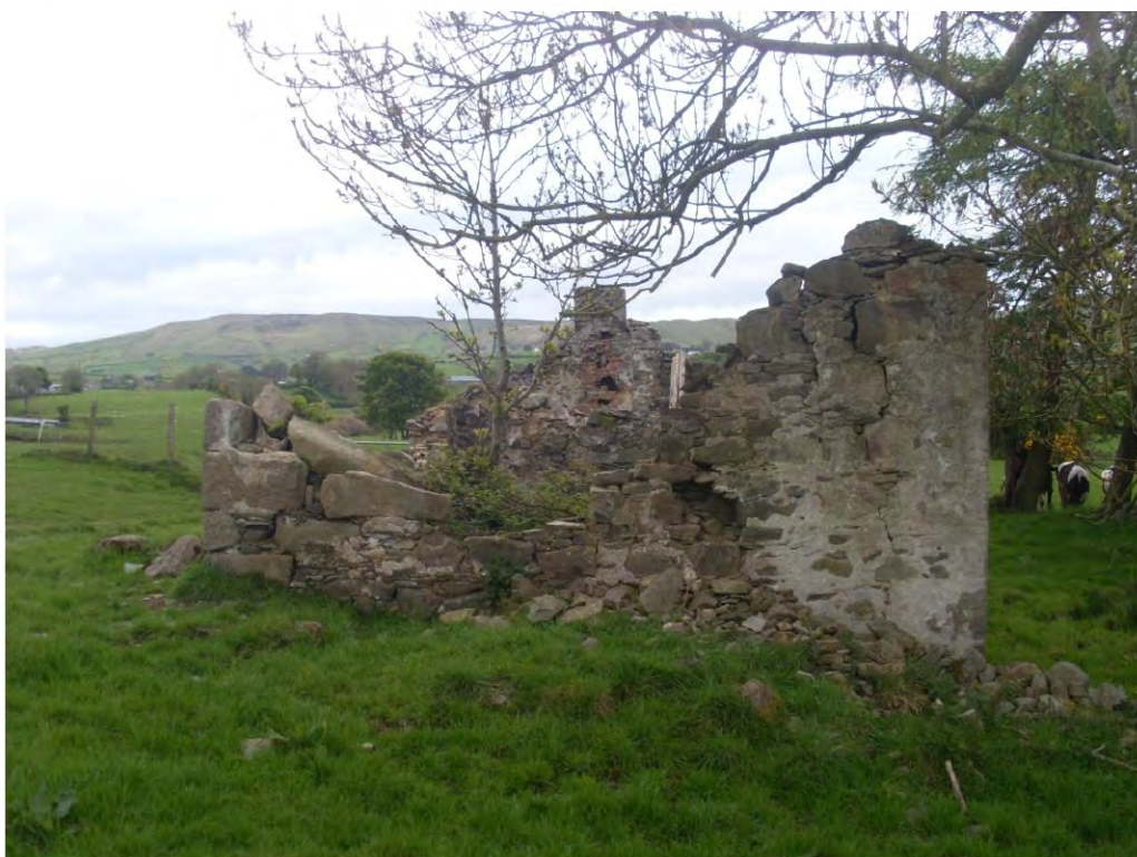
The north gable wall could not be described as being 'substantially intact'
