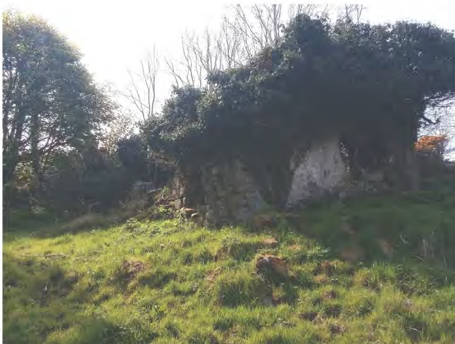
Image 4 Gable at North intact, South gable tumbled
