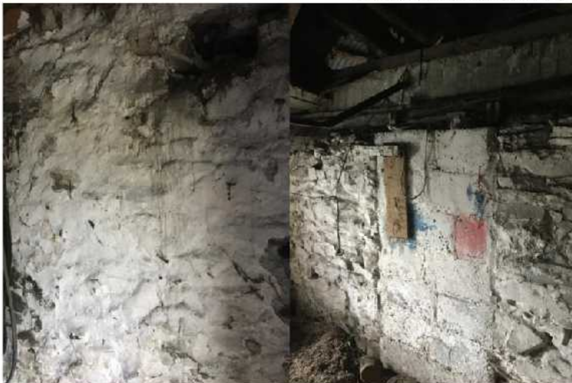
Photo 19 & 20 – Lime plastered internal walls and blocked up doorway between the two rooms
