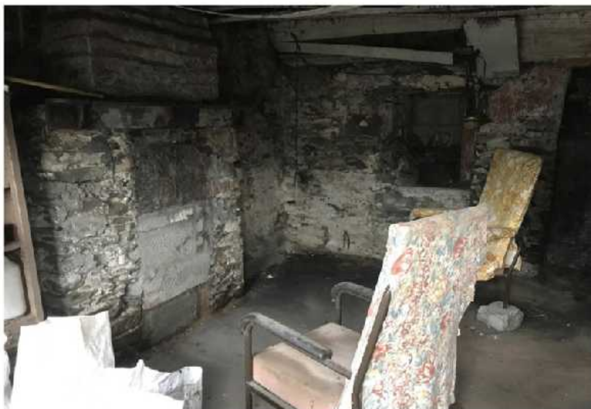
Photo 5 – Living room in former dwelling with blocked up fireplace, hearth, wooden mantelpiece, concrete floor, painted timber boarded ceiling, blocked up window and door openings to rear.
