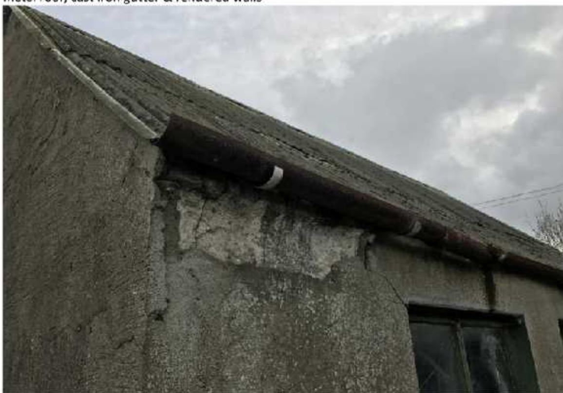
Photo 2 – North elevation detail featuring metal framed window, pitched metal roof, cast iron gutter & rendered walls
