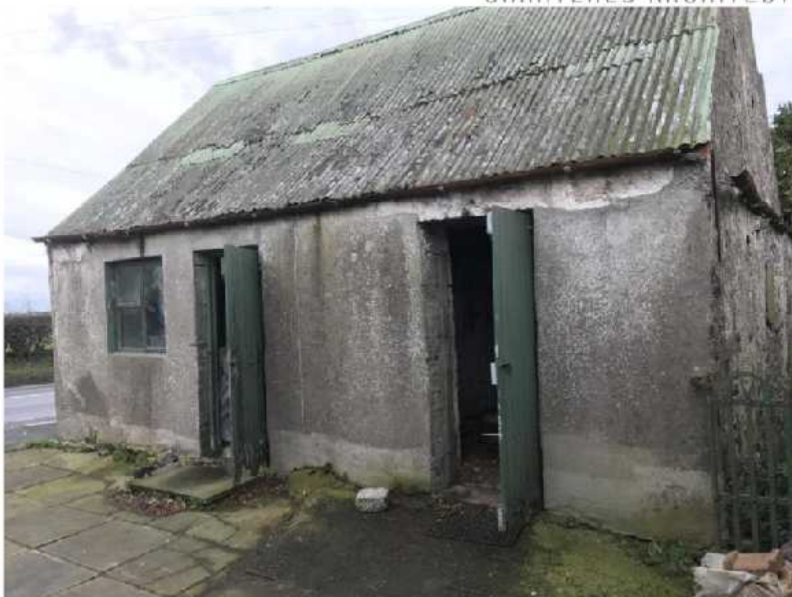
Photo 3 – North elevation featuring painted wooden doors, metal framed window, pitched metal roof, cast iron gutter & rendered walls
