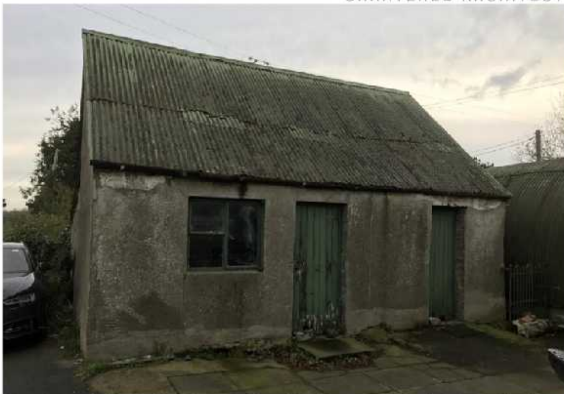
Photo 1 – North elevation featuring painted wooden doors, metal framed window, pitched metal roof, cast iron gutter & rendered walls
