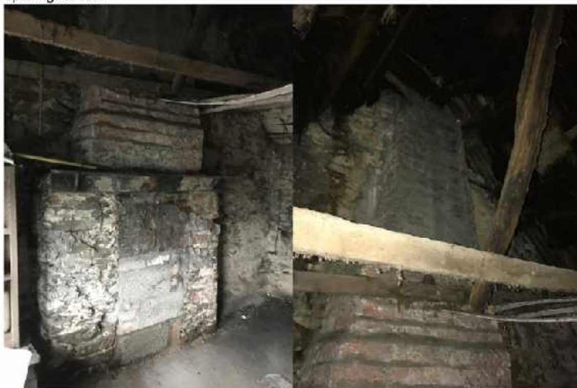
Photos 6 and 7 – Blocked up fireplace, hearth and chimney stack running up into roof
