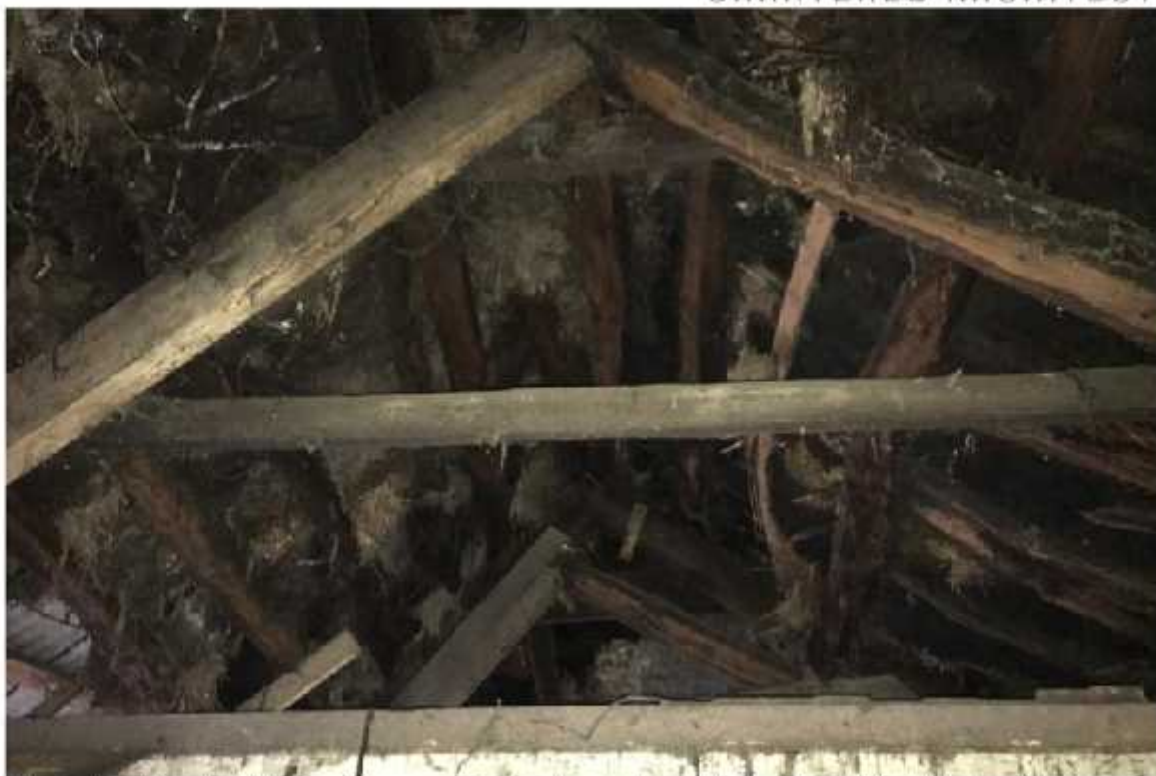
Photo 17 – Wooden 'A' frame truss with wooden purlins and remains of thatched roof
