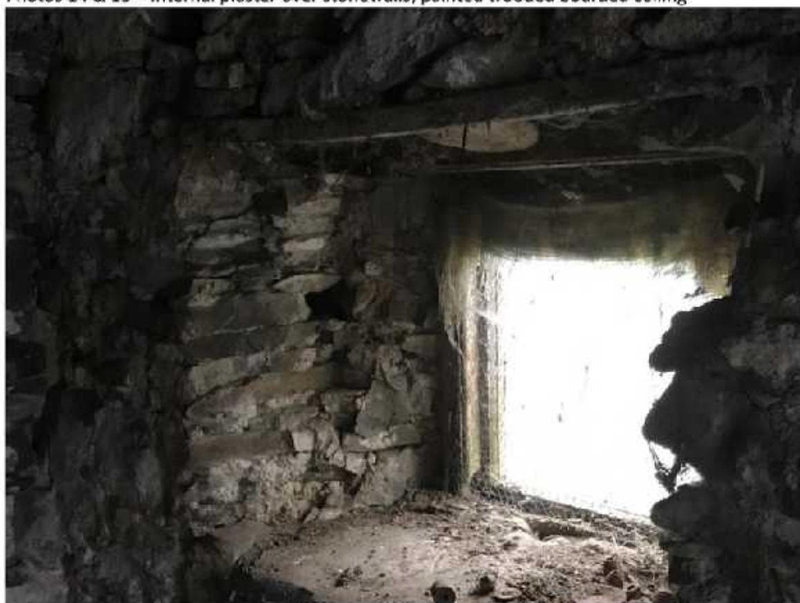
Photo 16 – Window opening to smaller room (former bedroom) with painted wooden window frame and wooden lintel
