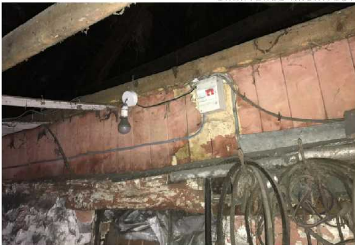
Photo 10 – Painted wooden panelling over connecting door showing power and lighting
