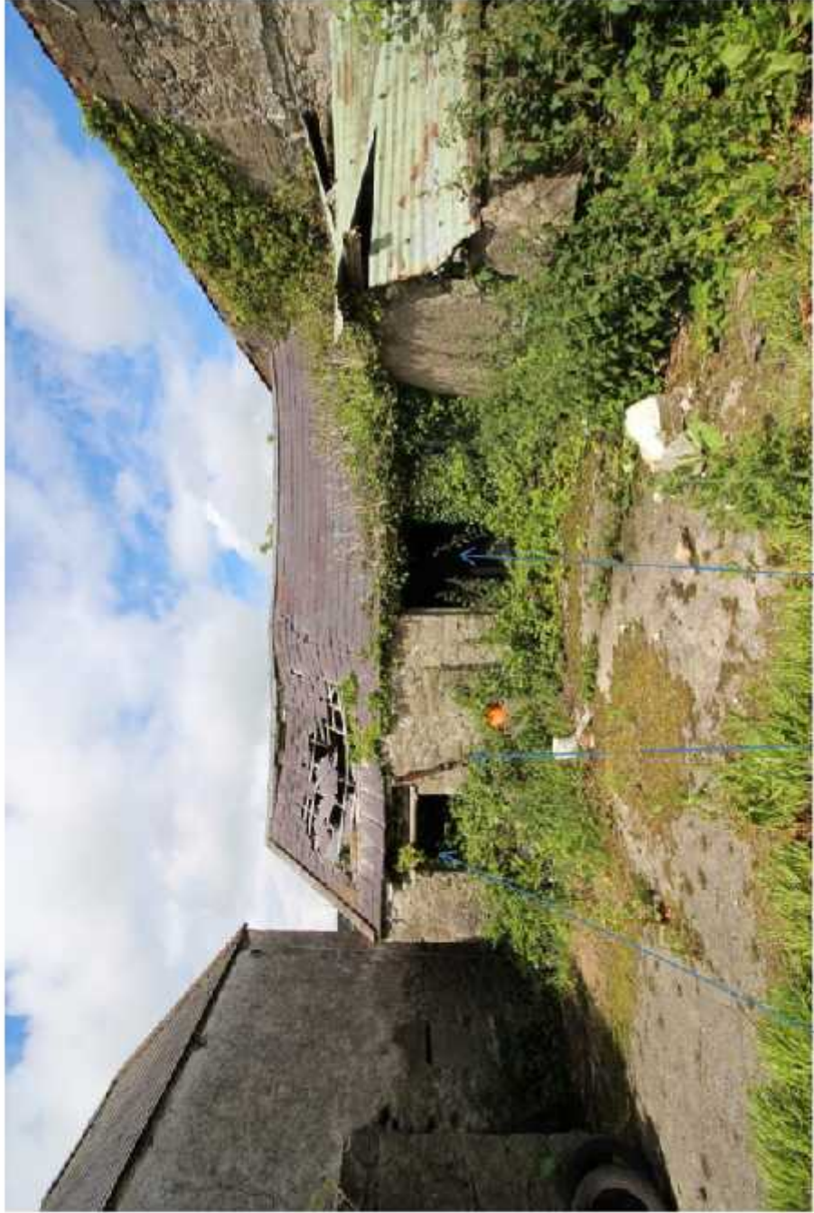
Domestic window and door openings to the front of the extended part of the house. Note the use of cast iron rain water goods, which is not consistent with agricultural use.
