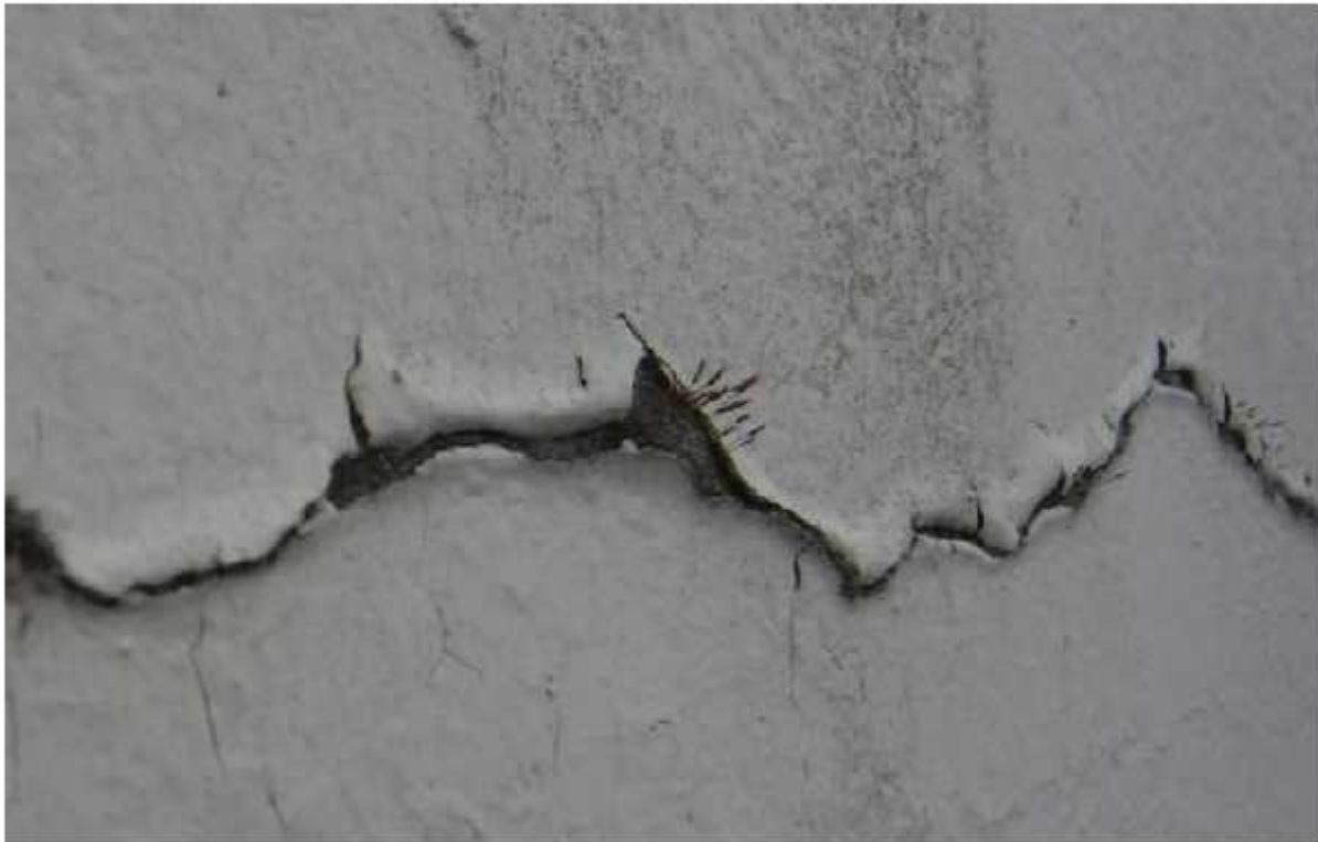
Figure 8 - Moss Growth was Observed Which may be Indicative of an Inactive (Dormant) Crack
